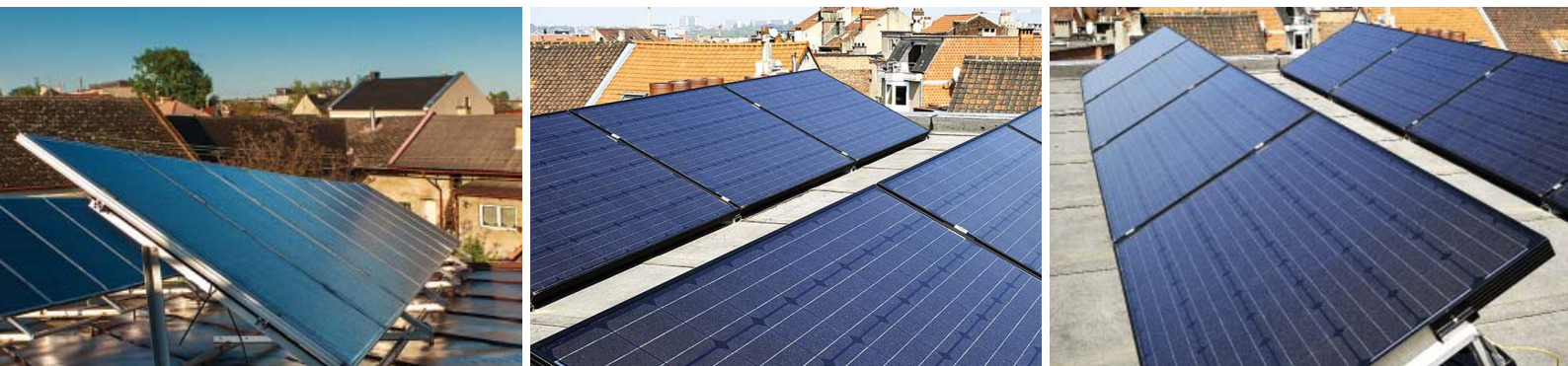
eVillage can combine private rooftops with a centralised PV area to optimize solar space
